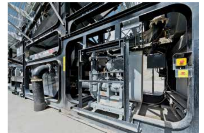
Centrifugal Pumps, Roll out for Service Access
